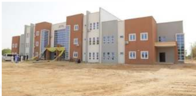
The Two-Story Academic Block at the Federal College of Education (Technical), Bichi Kano State.
